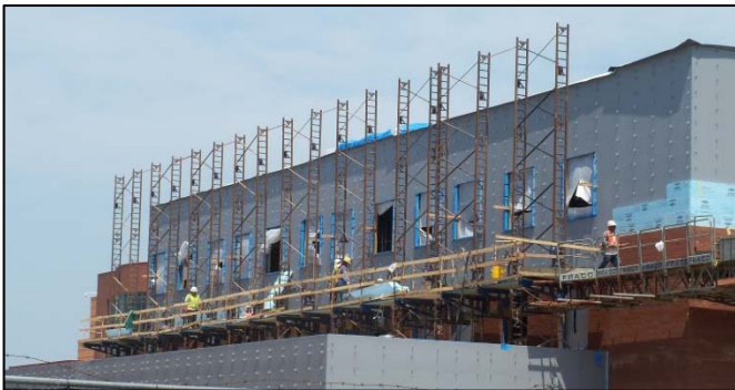
Figure 10 - View looking at southwest elevation. A MasonKing lift is required in areas where work is done above rooftops. These lifts have to be simultaneously cranked by hand to be lowered or raised. Personal photograph taken by Chris Pozza.
