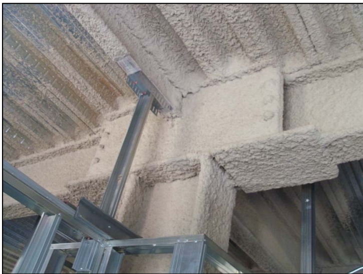
Figure 2 – Photograph of a Sideplate system (a moment frame that connects columns to beams and girders and can be single or double sided). Spray-on fireproofing has already been applied to the structural steel at this point of construction. Personal photograph taken by Chris Pozza.
