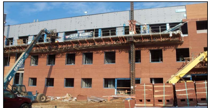
Figure 11 - View looking at east elevation. Fraco Lifts are used around exterior to provide efficient flow of construction along a large percentage of elevation at a time. Materials are lifted into place with a boom lift. Personal photograph taken by Chris Pozza.
