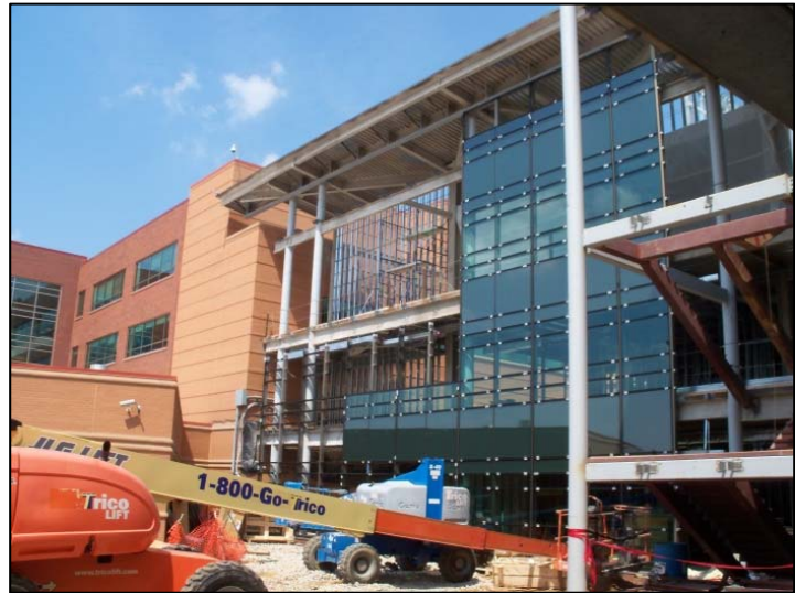
Figure 12 - View of west elevation curtain wall system under construction. The boom lift used during construction of the façade system can be seen at the bottom of the photo. Personal photograph taken by Chris Pozza.
