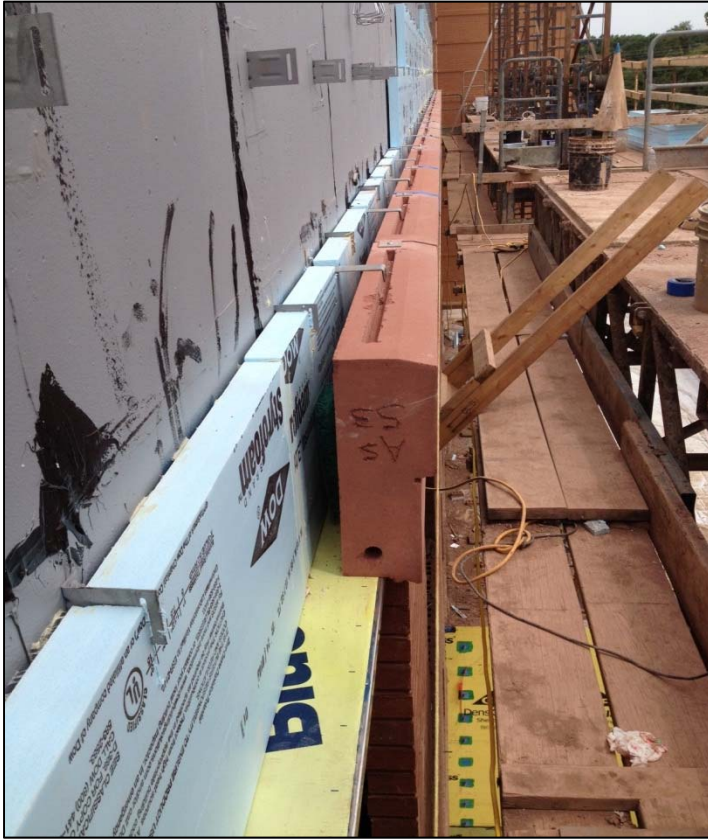
Figure 6 - Precast concrete can be seen above which make up the accent band along with east elevation. Personal photograph taken by Chris Pozza.
